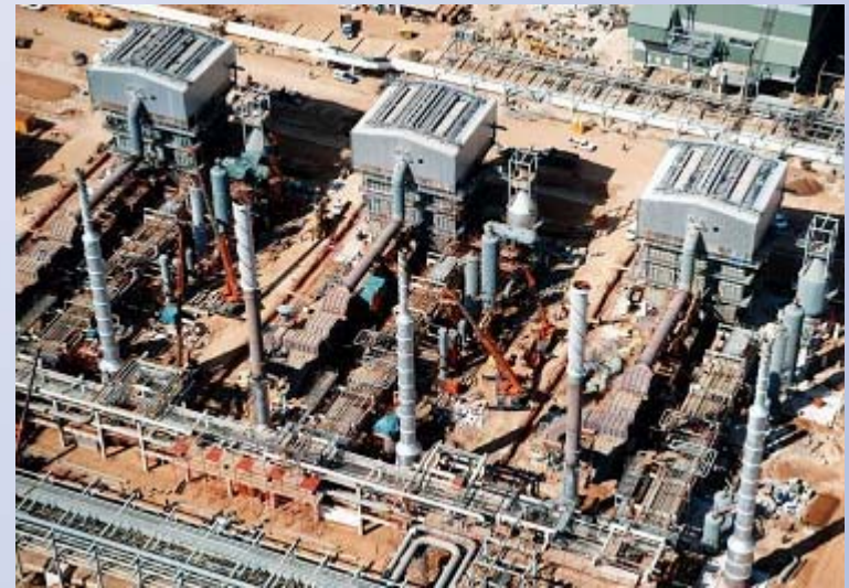
Combined Reformer, Moss Gas, South Africa
